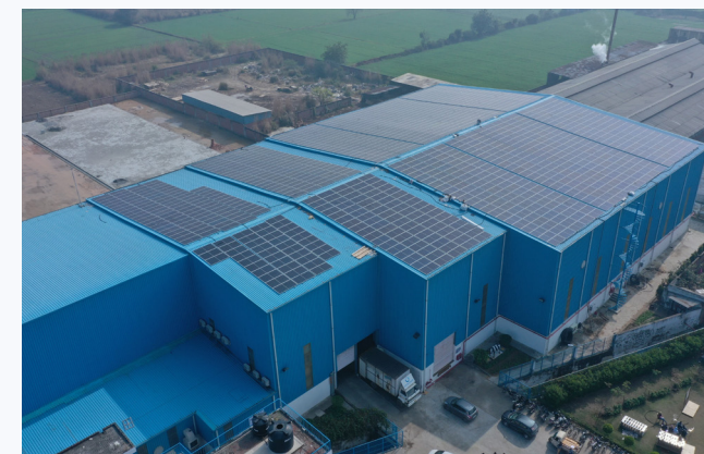
Warehouse and distribution center with solar panels LPS Bossard in Rohtak, India
