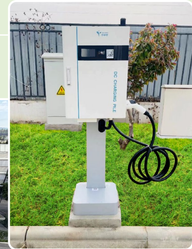
New charging stations: Bossard China – One of the four newly installed charging stations
