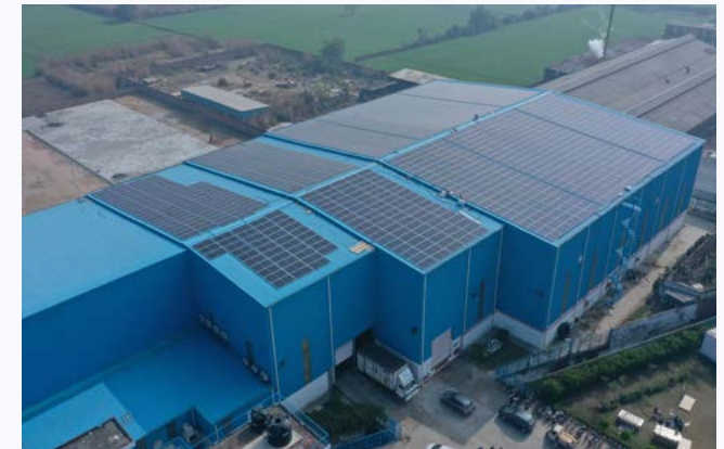
Warehouse and distribution center with solar panels LPS Bossard in Rohtak, India
